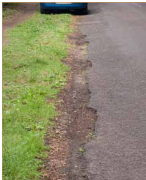
Damaged road edge
