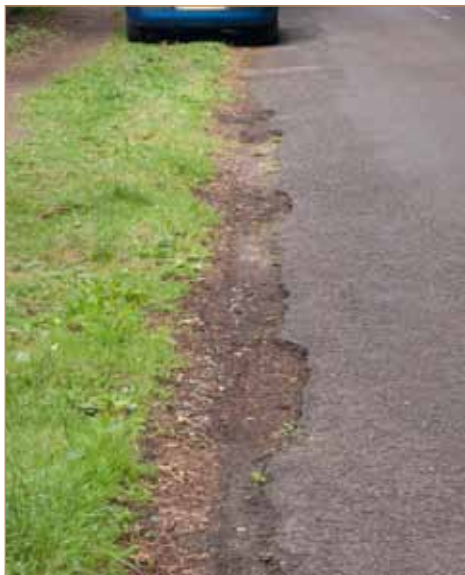
Damaged road edge
