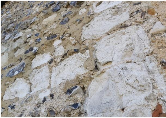
Fig 11 – Spalling ashlar stone on the north elevation.
