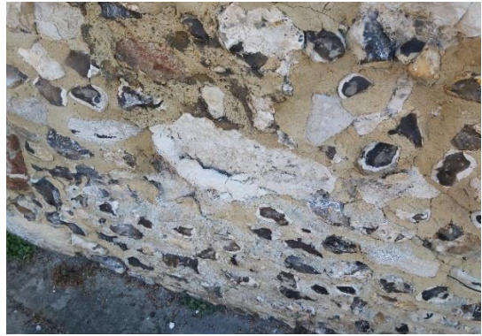
Fig 12 – Spalling ashlar stone on the north elevation surrounded by cement pointing.
