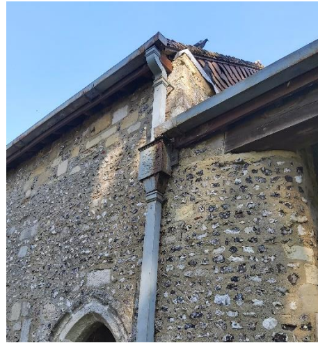
Fig 8 – Corroding hopper on the south elevation
