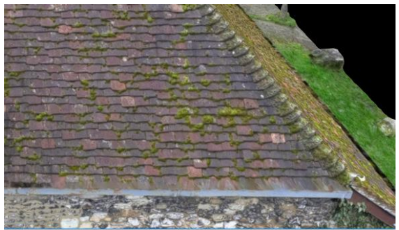
Fig 6 – Photogrammetric image of the same roof irregular tiling courses indicating failed fixings or battens.
