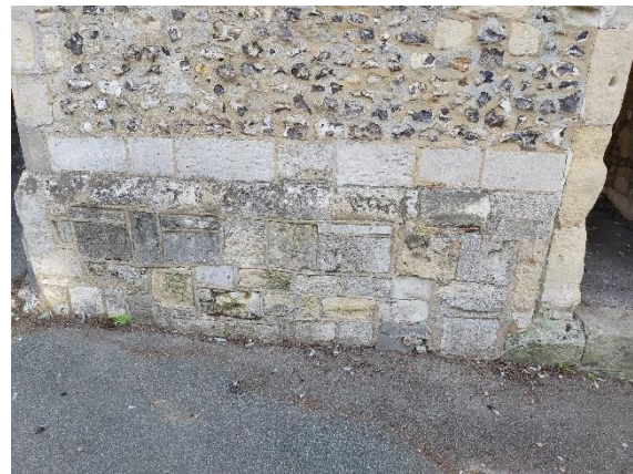
Fig 10 – Unsightly cement strap pointing and pointing around flints on the south elevation.
