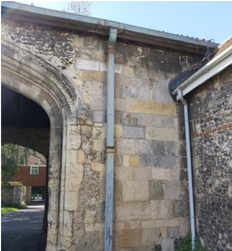
Fig 7 – Corroding downpipe on the north elevation
