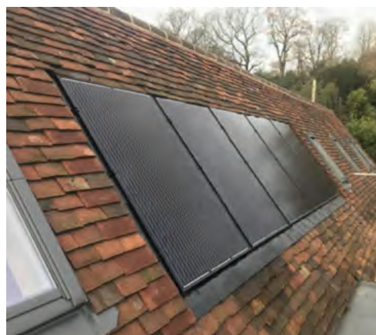
Photo 42. Solar Photovoltaic panels in a regular pattern and recessed into roof tiles.
