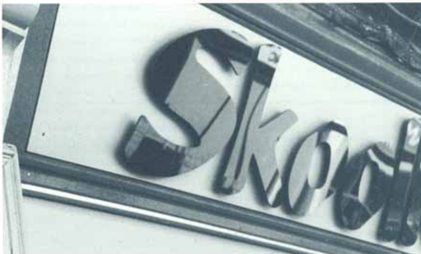
Inappropriate mounted plastic lettering can appear out of place when on an older building.
